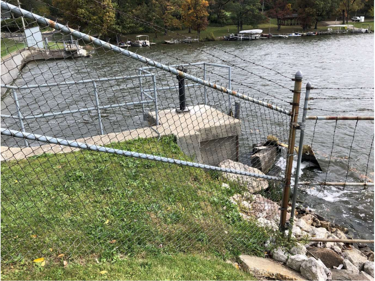
Photo 9: West Sluice Gate Control
