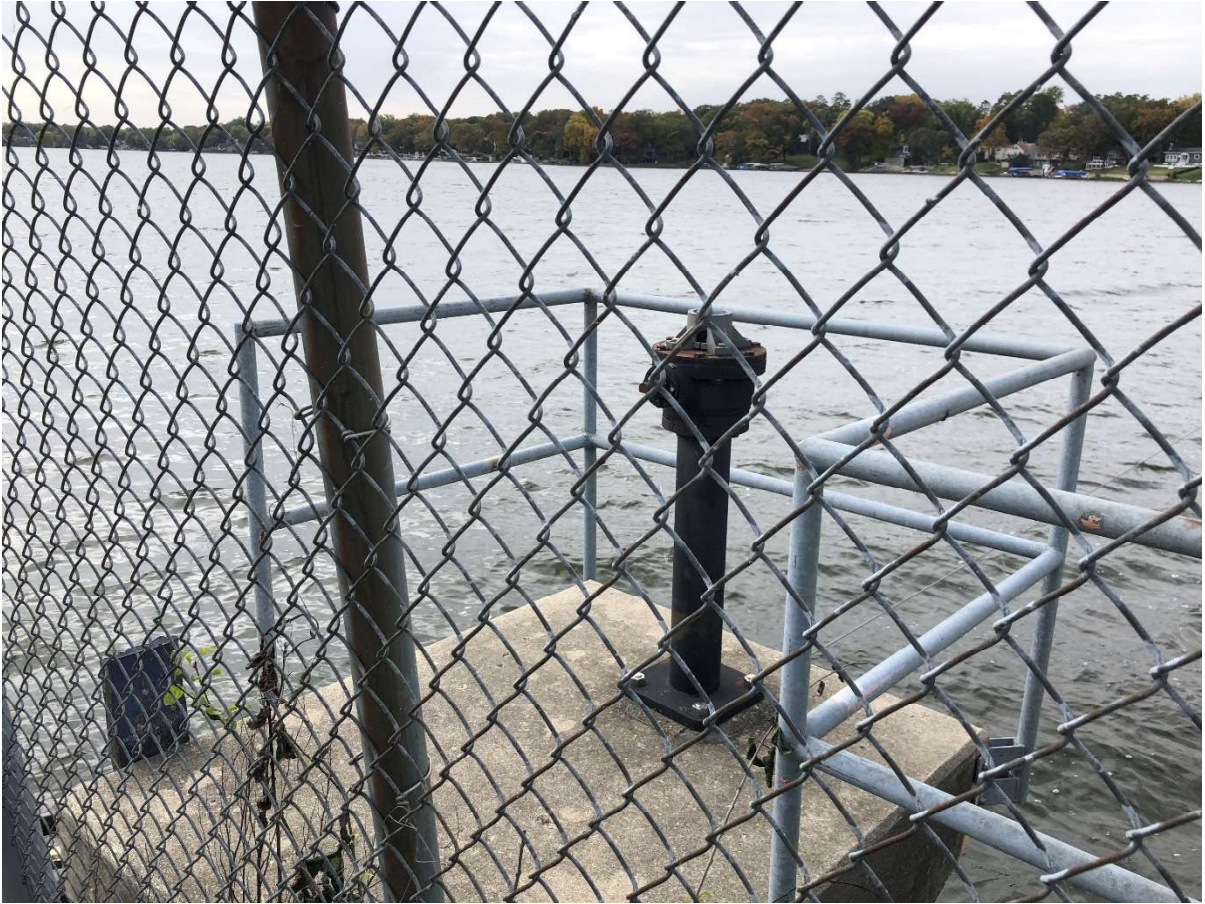
Photo 8: East Sluice Gate Control
